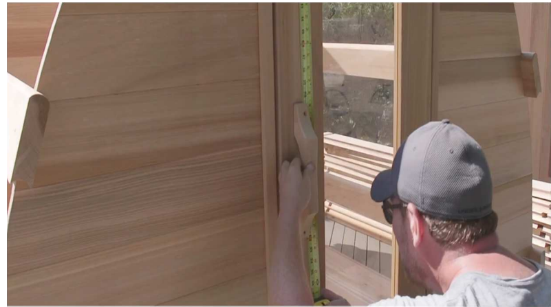
20. Measure the center of the door and attach the door handle using 2" screws.
