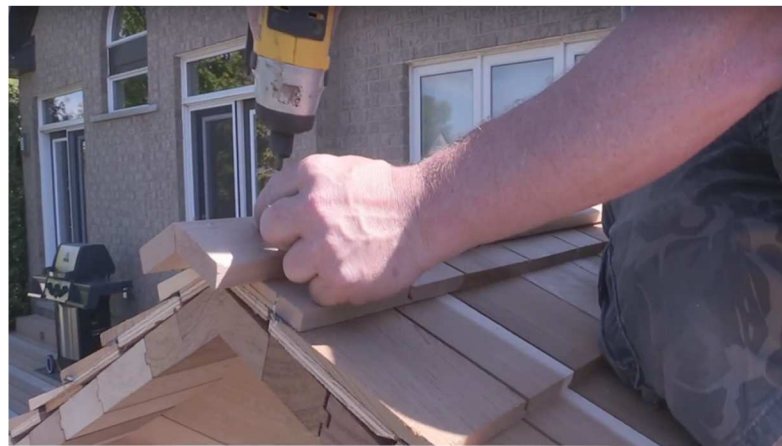
41. Screw roof ridge into place with 2" screws. (Approximately 1" overhang on each end)
