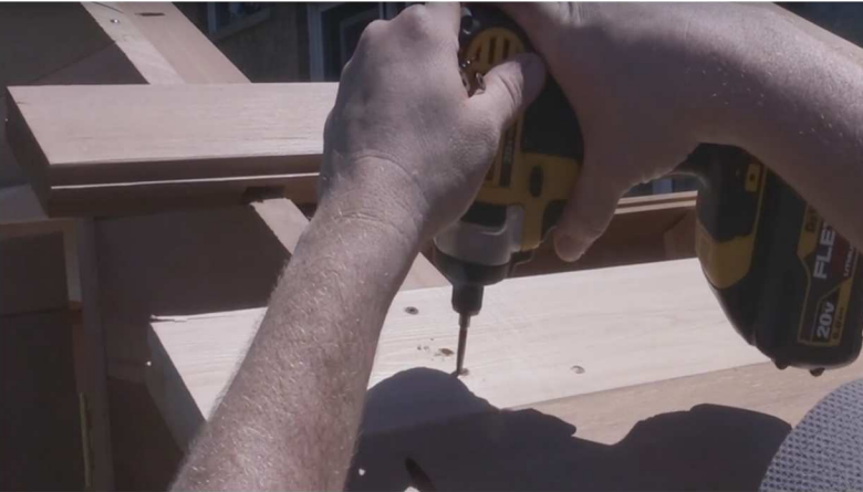
31. Secure overhang roof piece in place with 2 1/2" screws at either end and in center making sure the screw goes into center support.
