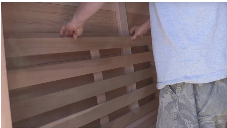
59. Screw back bench rest at ends through spaces in same manner as bench seats using 1 1/2" screws.
