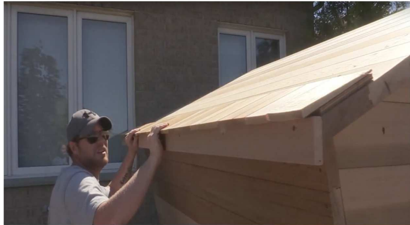
36. Start cedar roof shakes with 1" overhang at bottom and fasten to roof staves with 1 1/2" screws.
