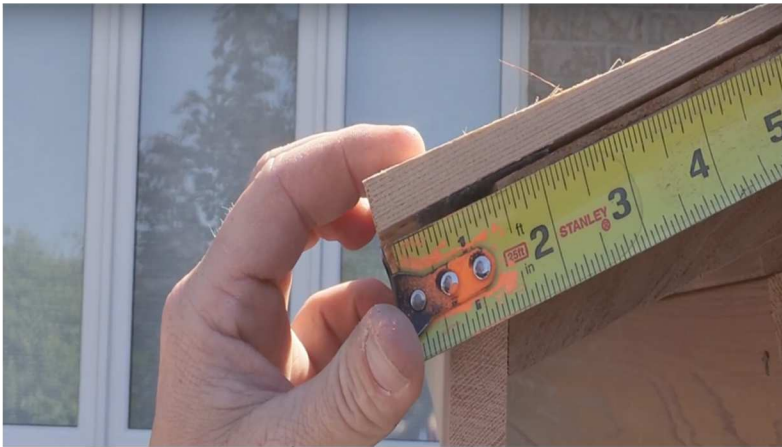
37. Start cedar roof shakes with 1" overhang at bottom of roof and fasten to roof staves with 1 1/2" screws.
