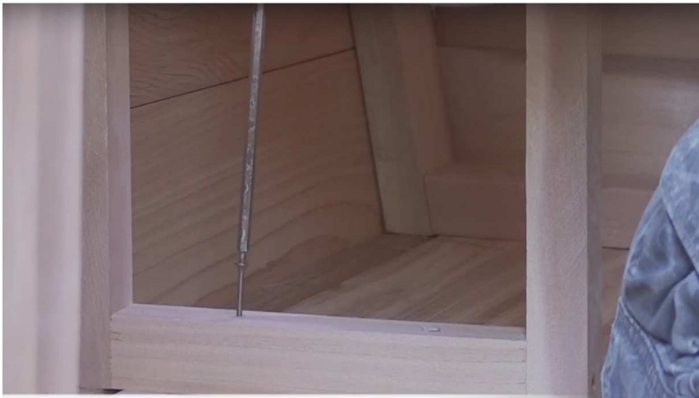
55. Screw support into floor using 2 1/2" screws, level bench and screw wall support in to front and back wall of sauna with 2" screws.
