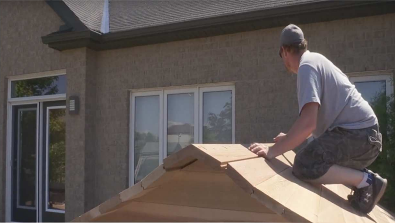
33. When placing peak piece in at top, there will be a slight bulge. Use a mallet to "finesse" these pieces in to fit correctly.
