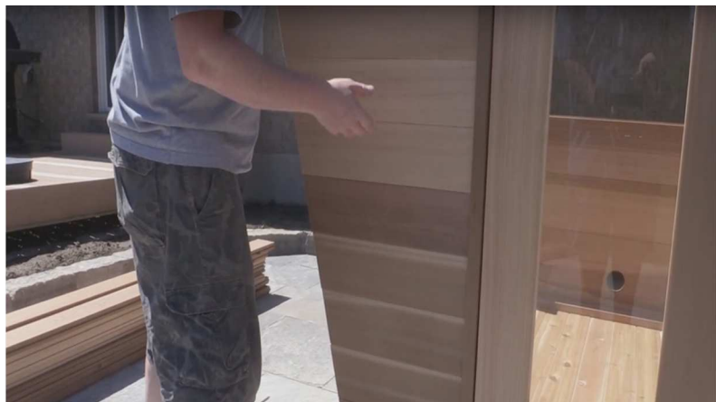
12. Screw wall support to bottom and to side in pre drilled holes using 2 1/2" screws.
