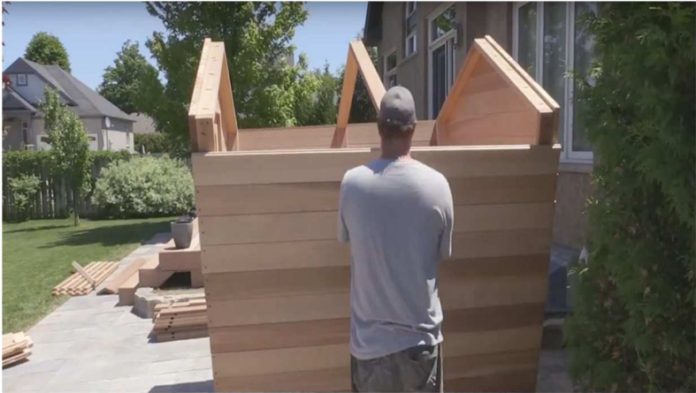
26. Continue to build wall upwards fastening 2 1/2" screws into staves at ends and middle support as stated before.
