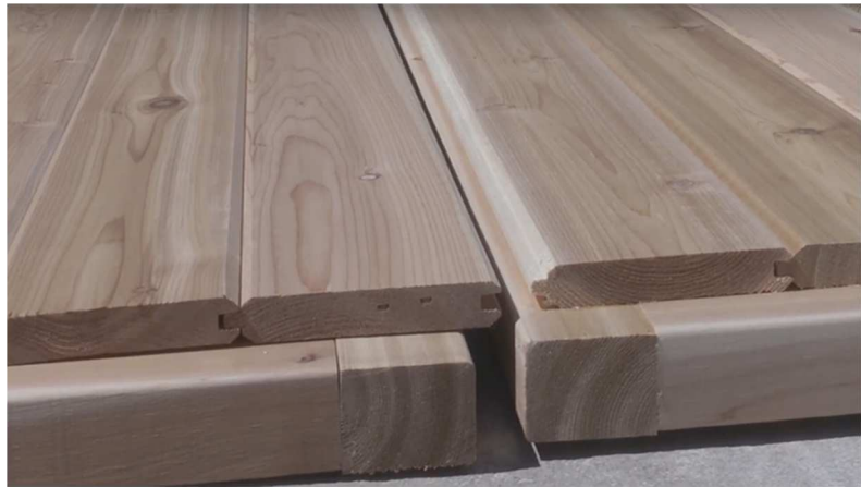
2. Slide tongue of 1 side into groove of other half. Make sure pieces are flush at both ends.
