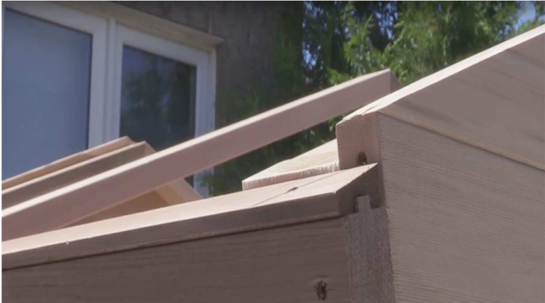
28. There will be approximately 1" distance from finished wall. This gap is intentional.
