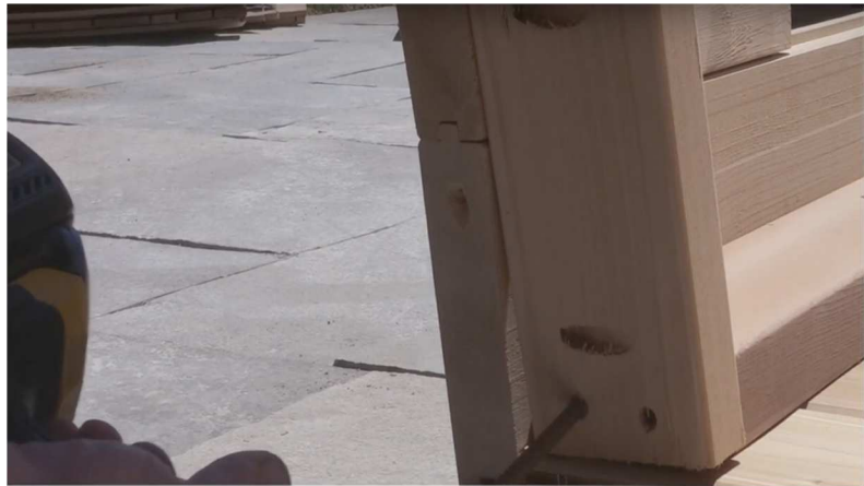
8. Screw wall support to bottom and to side in pre drilled holes using 2 1/2" screws.
