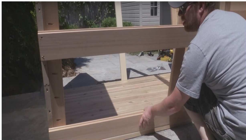
21. Starting at bottom of wall, fasten wall stave to end walls using 2 1/2" screws at either end and into middle support.
