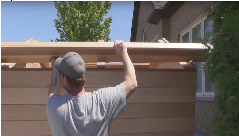
29. Square up roof overhang with sauna and tap notches into walls of sauna.
