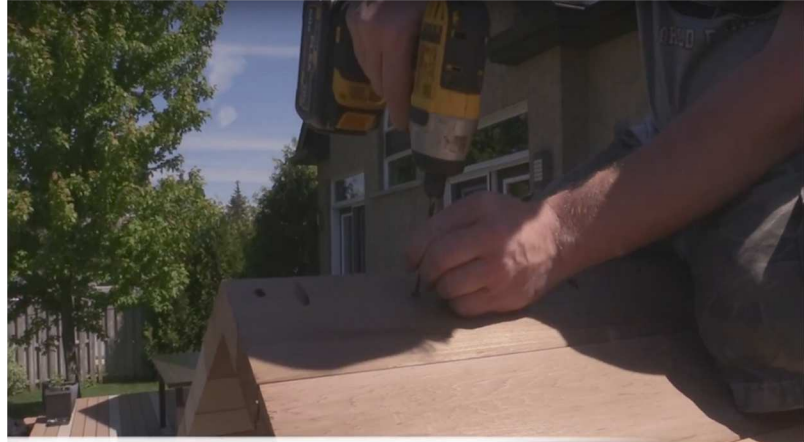
34. Screw roof staves in place at either end and into middle support with 2 1/2" screws.
