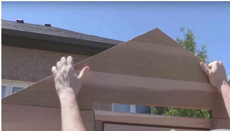
15. Attach front wall, fasten from wall support and top on both sides using 2 1/2" screws.
